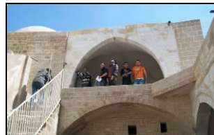
Figure 10: Stone renovation of the southern facade of the first-floor iwan (before and after).
